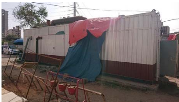
1.2 MW Gas Genset at ZU Clifton Site
