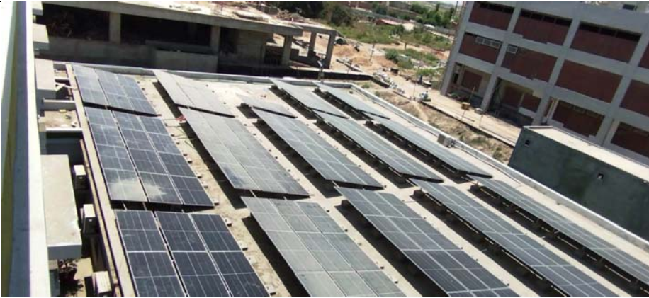
Renewable Energy: Solar System to minimize Electricity consumption
