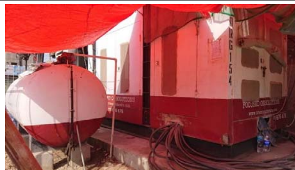
1250 KVA DG Set at ZU Clifton Site
