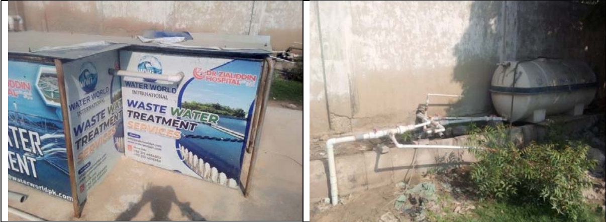
Example of Sewage Disposal Treatment at Ziauddin University
