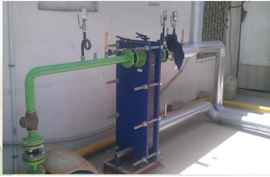
Co-Generation Hot Water Supply
