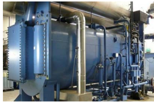
2x300 Tons Absorption Chiller
