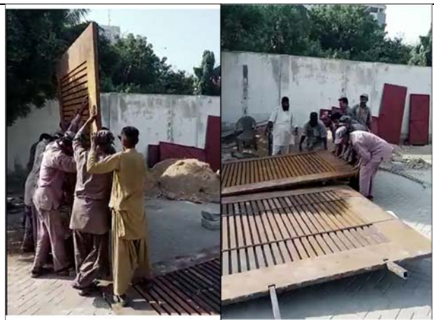
University Main Gate Installation
