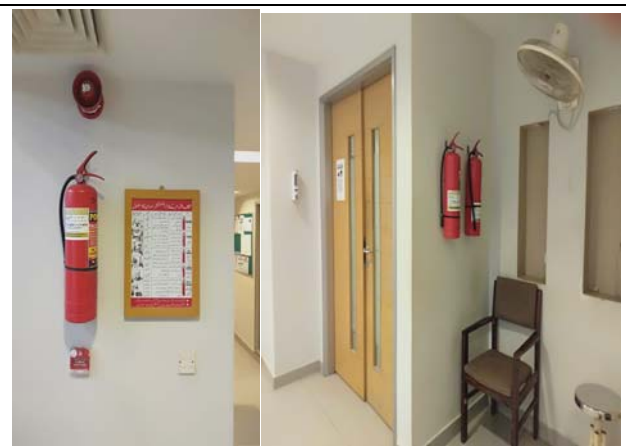
Fire Extinguisher System
