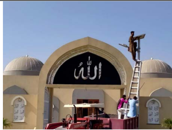
Solar Street Lights at Link Road Site
