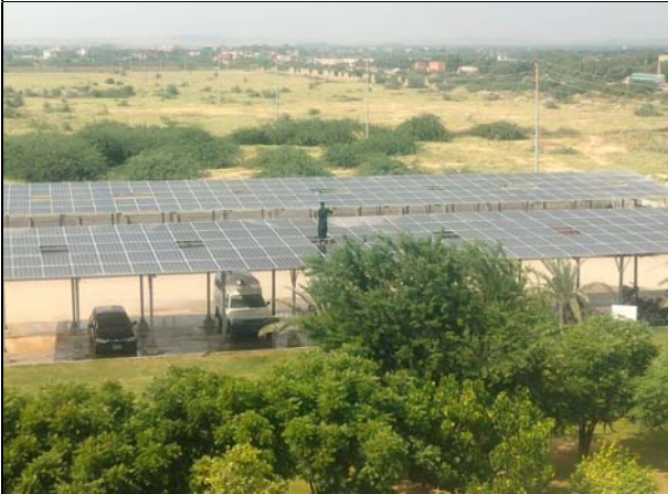
Solar Parking at Link Road Site
