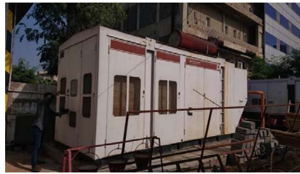
725 KVA DG Set at ZU Clifton Site
