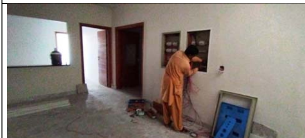
Maintenance of Building Wirings
