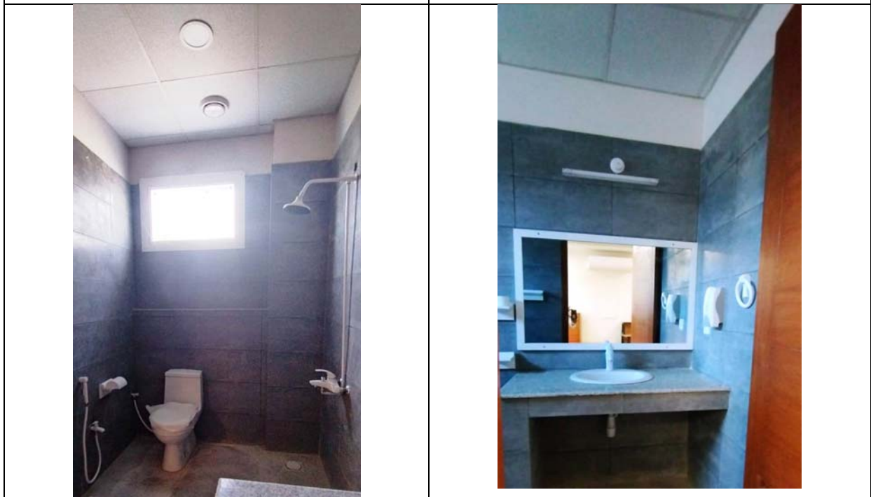
Example of Wastel/ wash basin, Hand Dryer & Soap Dispenser
