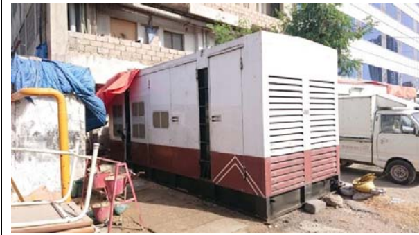
750 KVA DG Set at ZU Clifton Site
