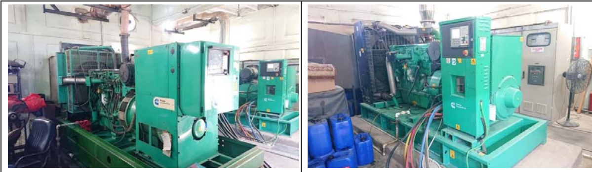
500 KVA two DG Sets at ZU Clifton Site for Backup
